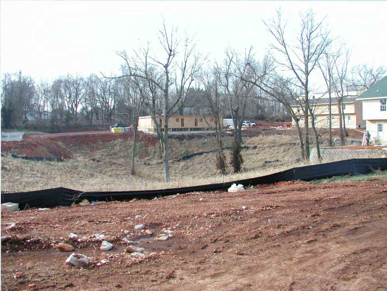
Sinkhole in residential development on SE corner of Kansas Expressway and Walnut Lawn, Springfield, MO
